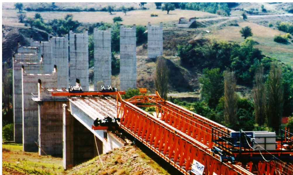
View of railway track construction works on Kumanovo – border with Bulgaria railway section, the former Yugoslav Republic of Macedonia.
