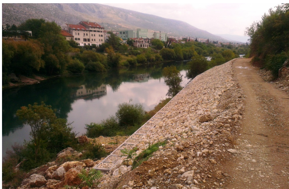
Neretva river embankments and location of future collectors, Mostar, Bosnia and Herzegovina.
