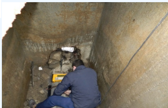
Ultrasonic flow meter installed to the inlet pipe of District Metering Area
