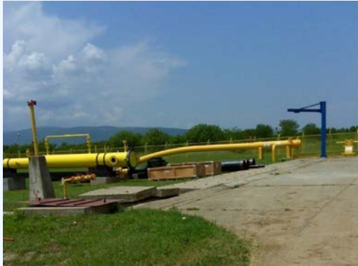
Gas Measuring Station
