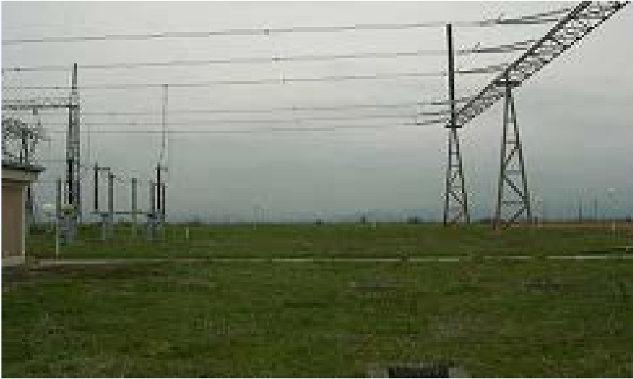
SubStation (SS) Bitola 2 (OHL starting point) view toward the proposed OHL corridor
